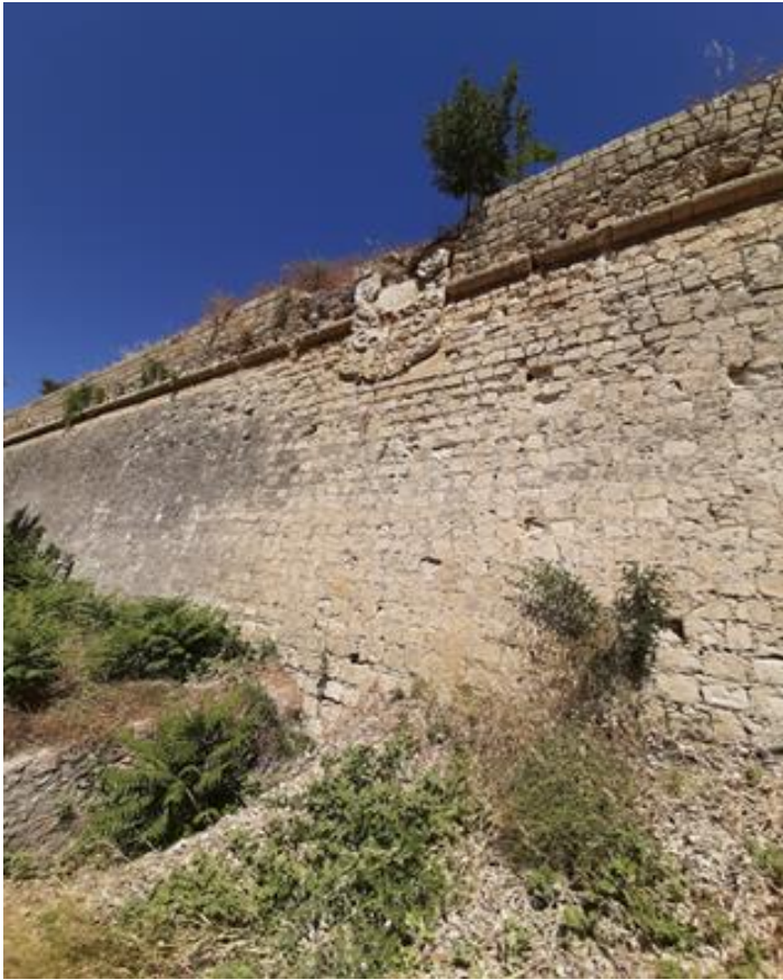
Figure 2. Photo of a part of the Heraklion City Walls in Crete (Photo credits: NTUA).
